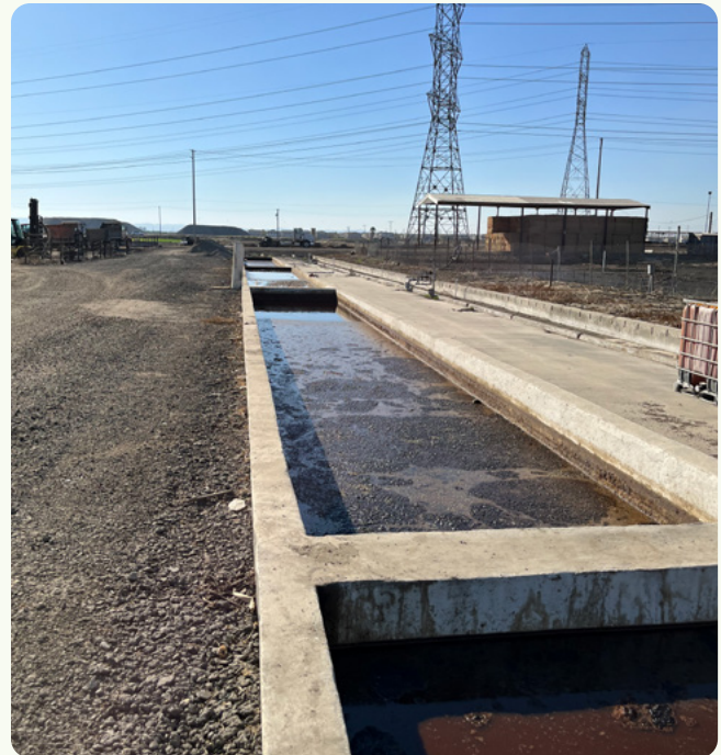
Beginning of anaerobic digestion process before being converted into energy source.
